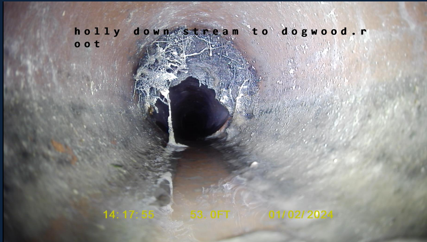
Bottom Right: Approximately 65% blockage caused by roots in a section of pipe that requires multiple visits per year to keep clear. This section of pipe has been submitted as part of our relining/repairing project.
