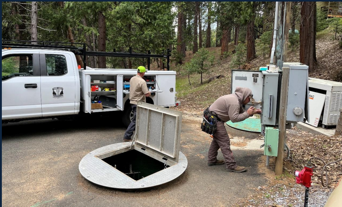
Left: Curtis Smithers and Robert Smith replacing 3 failed floats. This type of work was done by contractors in the past but can now be done by THCS D due to Curtis’s previous background in the sewer industry.
