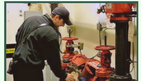
All shifts have completed the annual Group R fire inspections, covering three commercial residential occupancy units.
